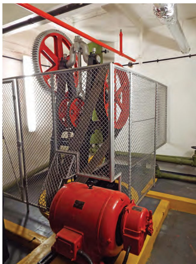
Disused pump in Australia House used for water abstraction. Photo John Lill
